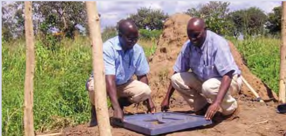
Edward Bwengye-Kahororo (right) with a district water officer constructing a temporary latrine for flood-affected primary school pupils
