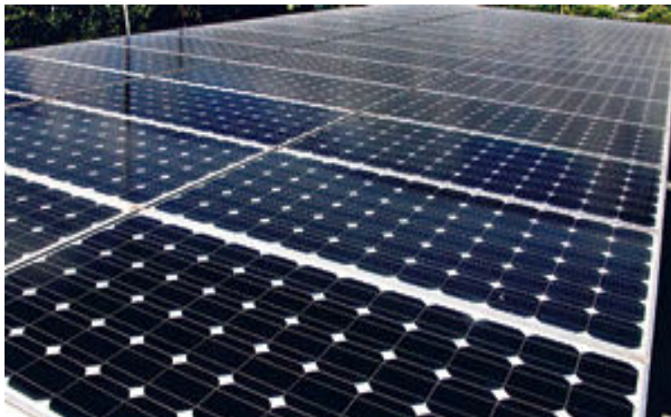
The array of solar panels on the Nikini building rooftop
