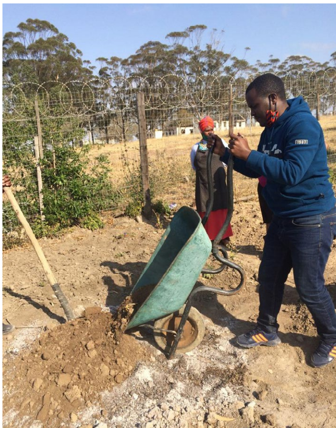
Sidney working with local community members to construct vegetable tower gardens for households and ECD sites.
